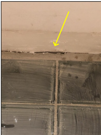
Glass block window in basement needs caulk
