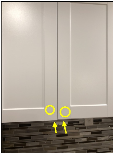
Doors out of line and missing knobs.
