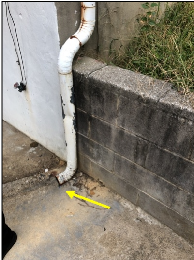
Downspout end crushed
