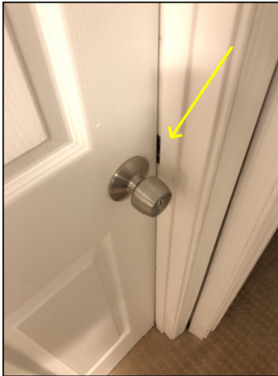
Door does not latch shut
