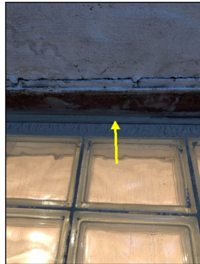
Window in storage area under deck needs caulk
