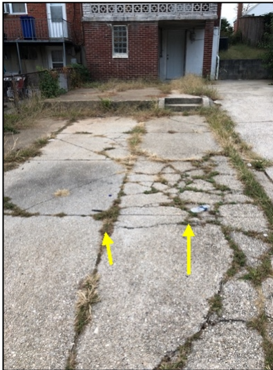
Cracked, plant filled driveway
