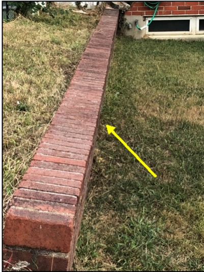
Retaining wall leaning
