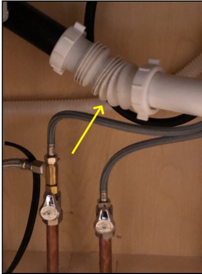
Flex drain under kitchen sink
