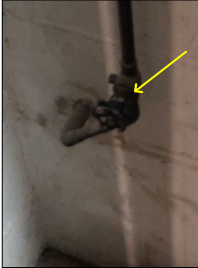
Leak at water main
