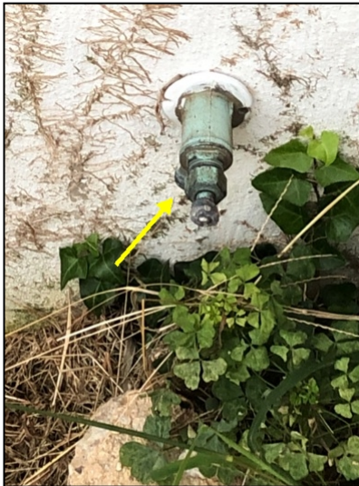
Front exterior faucet
