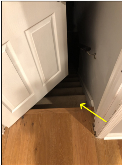
Basement door opens over stairs
