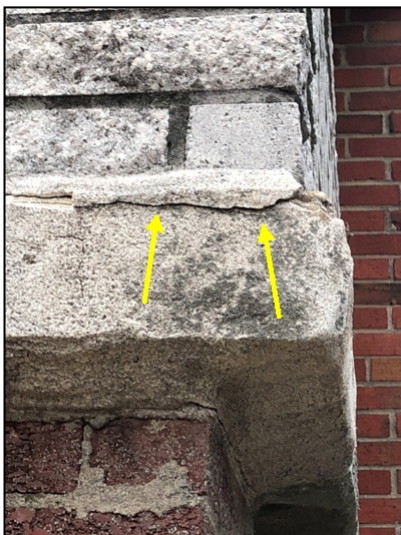
Cracking deck platform
