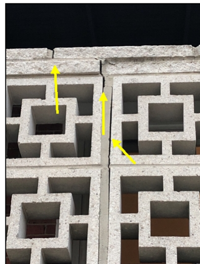
Cracking safety wall
