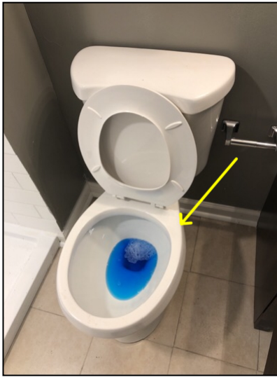
Loosely mounted toilet
