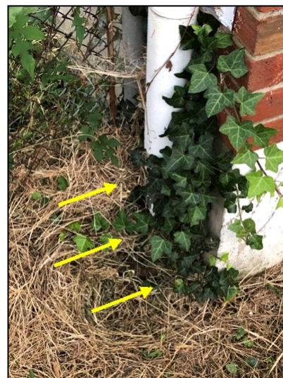
Weeds and vines around drain
