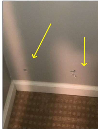
Holes in closet wall (front bedroom0
