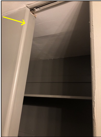
Bathroom closet second-floor missing door
