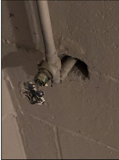
Large gap by rear exterior faucet
