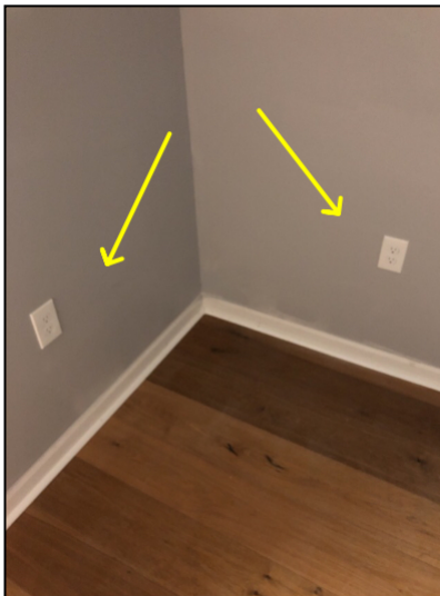
Open grounded outlets
