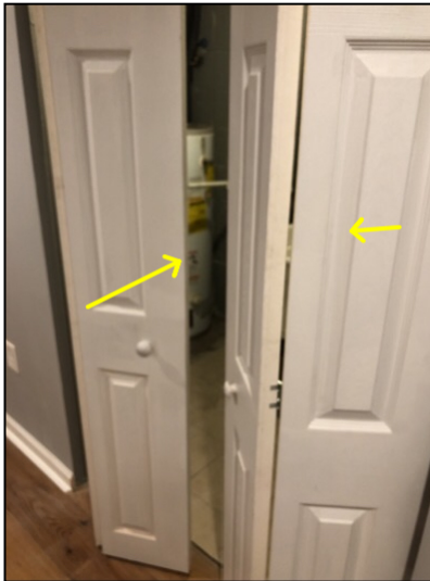
Heater closet enclosure doors
