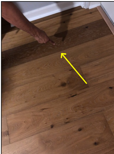
Weak spot in flooring
