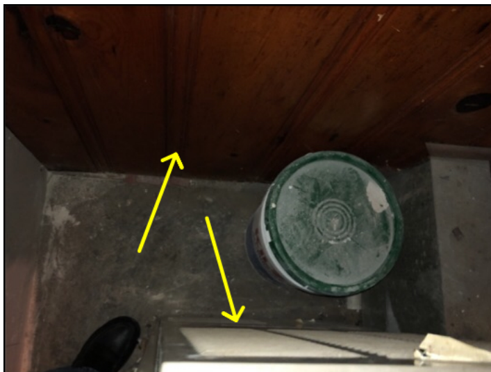
Are insufficient space between heater access and wall
