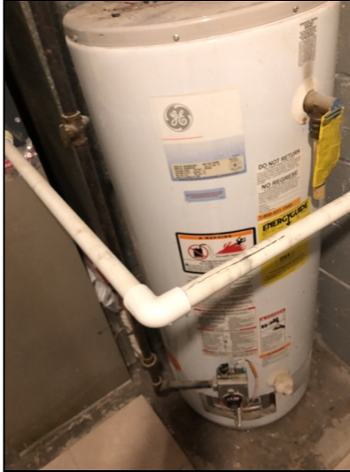
Inoperative water heater
